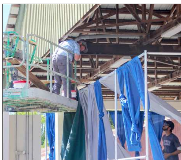
Crews work on last-minute adjustments Thursday to get ready for opening day of the Putnam County Fair.
